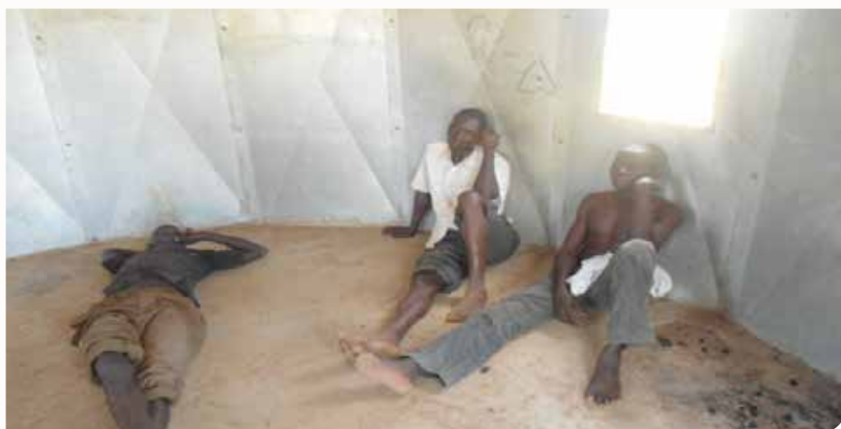
The window (above the inmate on the right) at Mucwini Police Post (Kitgum District) through which suspects dispose of human waste
