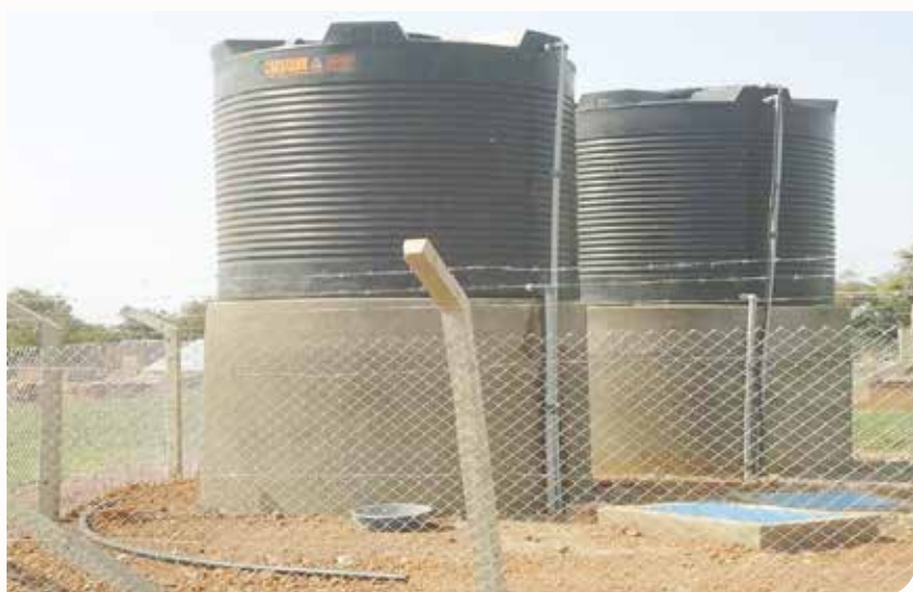
A water treatment plant constructed by Water Mission Uganda at Bukungu landing site for the residents.
