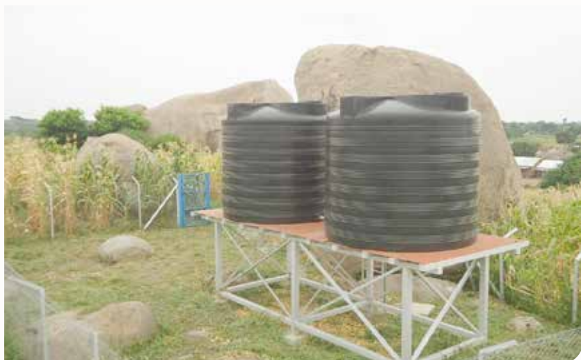
An enclosed water treatment plant at Lyingo landing site. It lacks security to safeguard the solar panels for the water treatment plant.
