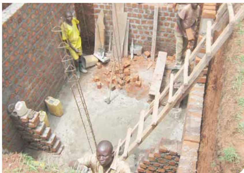
Construction of septic tank for water borne toilets at Ntenjeru Prison in Kayunga District
