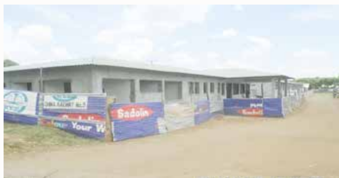
Construction and renovations taking place at Nebbi General Hospital in Nebbi District under a World Bank project
